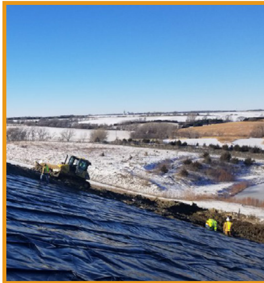
Pictured: Workers deploy the geomembrane cover on the landfill in Butler County
